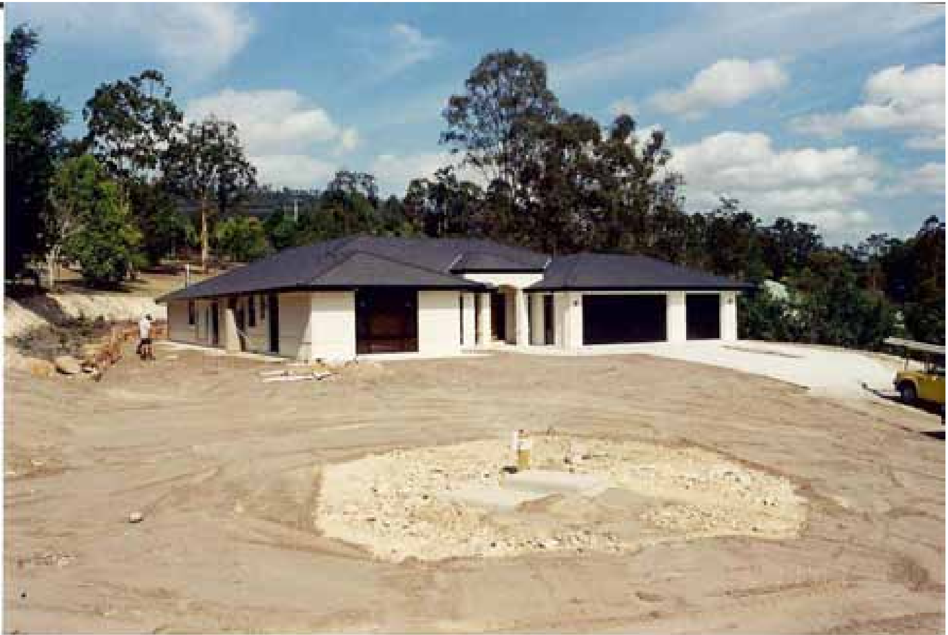
November 2001 - The house nears completion, natives are planted on the top bank and we have an exposed 'sewerage system' in the middle of what is to be the front lawn
