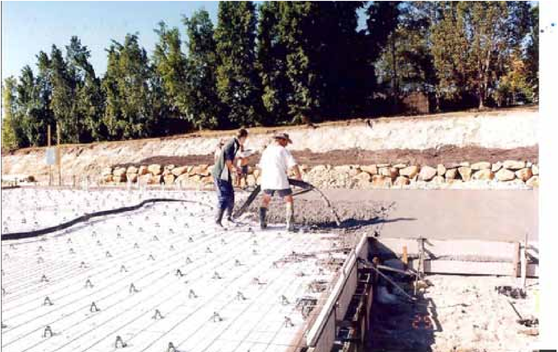
Finally we have the pad for the house laid and soil in the top retaining wall
